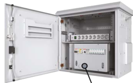
KGYS Electricity Distribution Unit Closed State
